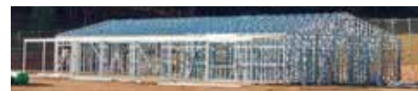
An update on the construction of a Multi-purpose Community and Relief Centre on Cox's Creek Road, which is well underway. The building is a direct result of the 2019-2020 Black Summer Bushfires and subsequent funding.
